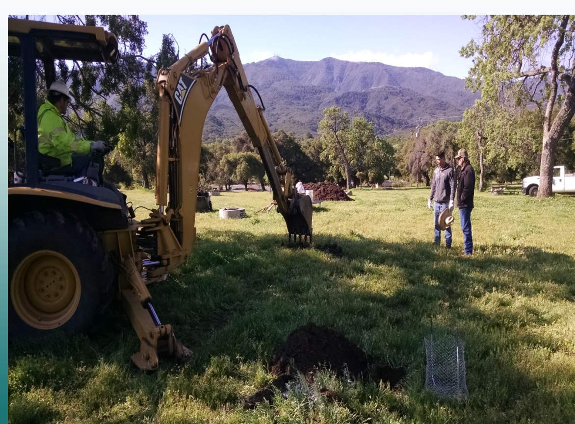
Use of a backhoe to dig rough holes for planting with a professional gopher cage.
